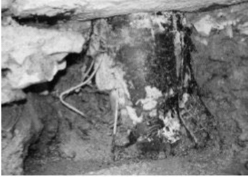
Photo 11.3. Damage to pile head
