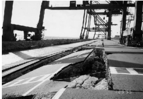
Photo 6.2. Liquefaction-induced flow behind a quay wall in Kobe
