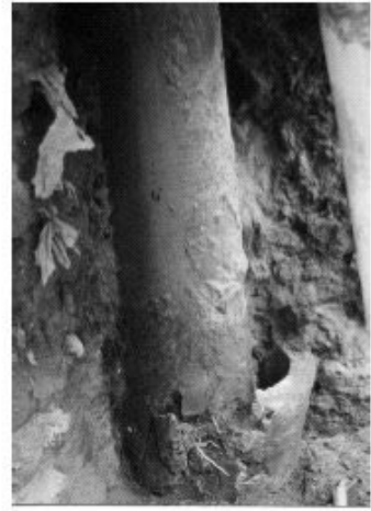
Photo 11.4. Damage to pile near ground water table
